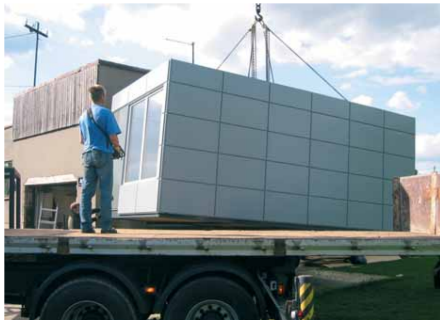
PROVIDING SOLUTIONS: Tomra Baltic signed an agreement to provide the Selver supermarket chain with 20 RVMs this year in Estonia. Three of the locations where these machines were to be installed however had difficulties finding the right spot to place the machines. Tomra Baltic then developed a special kiosk solution to house the machine, which is shown here being delivered and installed near the entrance to one of the Selver stores.
