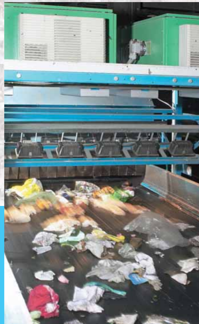
The waste material passes under the TiTech High Resolution Scanner at a rate of between one to ten tons per hour.
