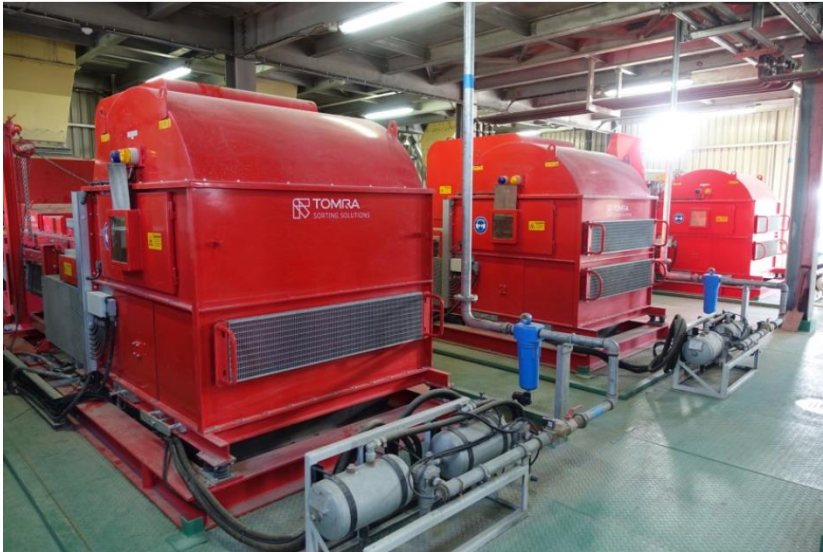
The TOMRA XRT sorters installed at the Karowe Mine in Botswana.
