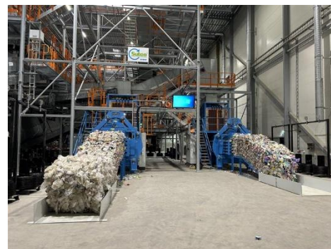
Finished Goods Baling
